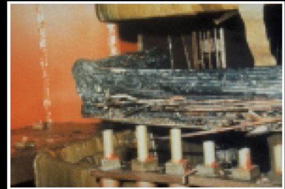
From left to right, the tan-colored paper on the upper winding is intact but burned out below. Next, paper is completely burned out to the right but not left. Last, copper strands have melted.
